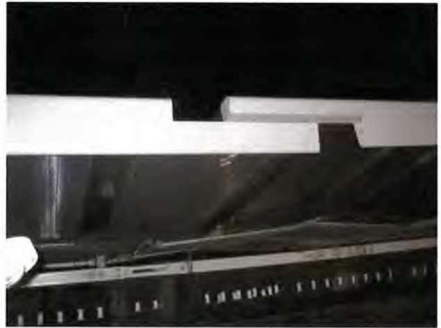
Figure 1: West Gate Bridge Barrier movement joint being installed. View from top of sliding top rail joint and overlapping mesh panels
