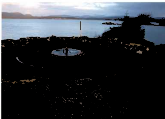
Generator for lyskastar.
