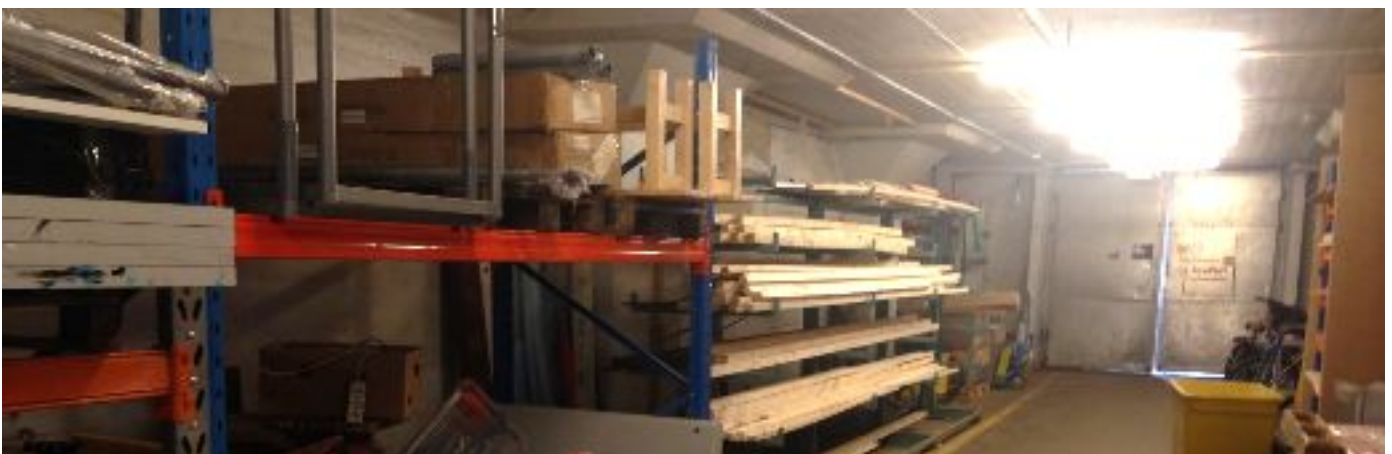
Original 1st Floor Storage of Khib that will become Gallery/Project Space. The Steel Doors that need to be replaced are in the center of the image.
