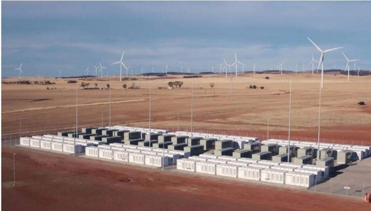
Tesla's 100-megawatt battery in Jamestown, Australia (Neoen / AFP)
